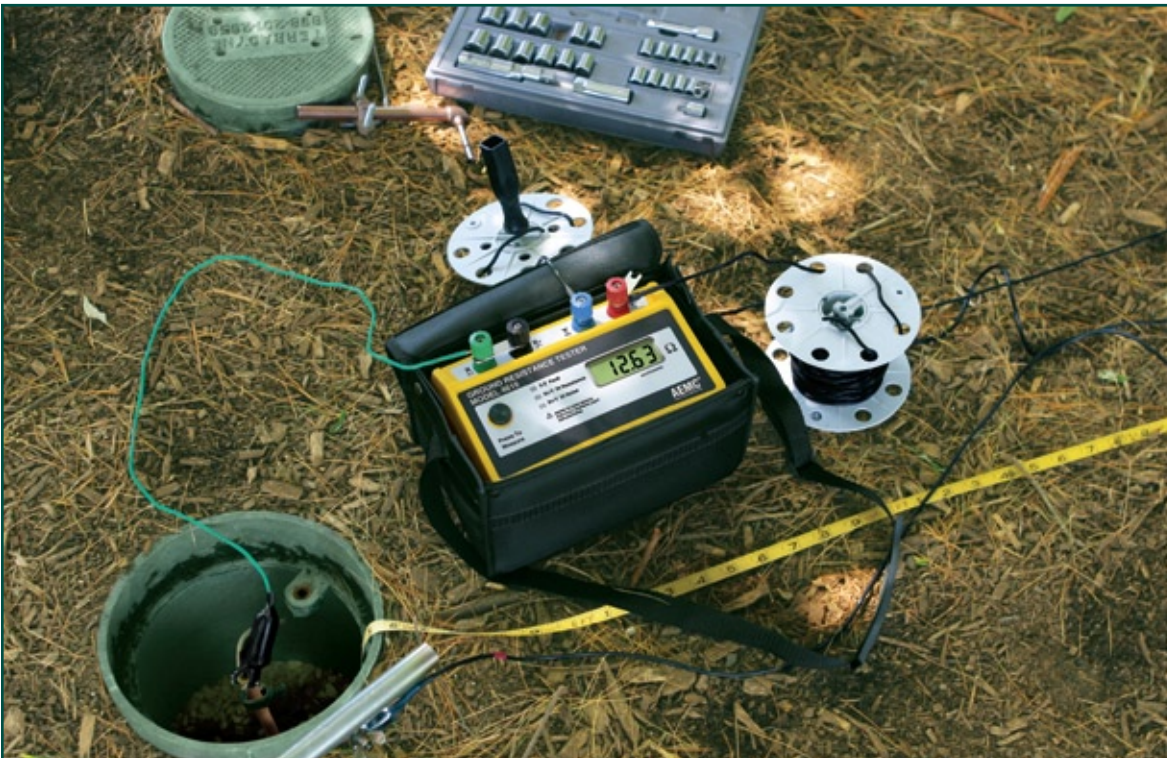
Ground Resistance Tester Model 4610 checks the ground rod using the Fall-of-Potential method.
