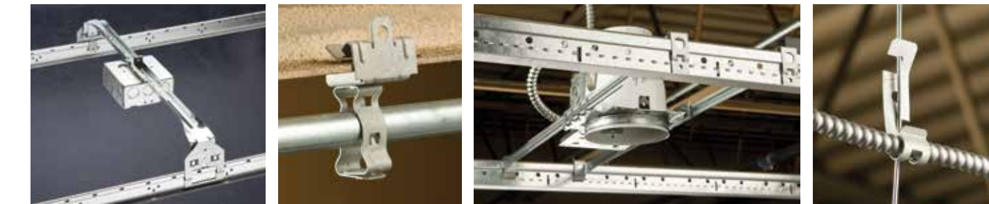
Electrical box from T-grid
